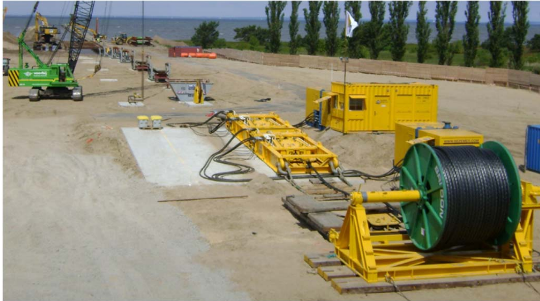
Figure 2.16: Typical Shore Pull Winch Configuration
