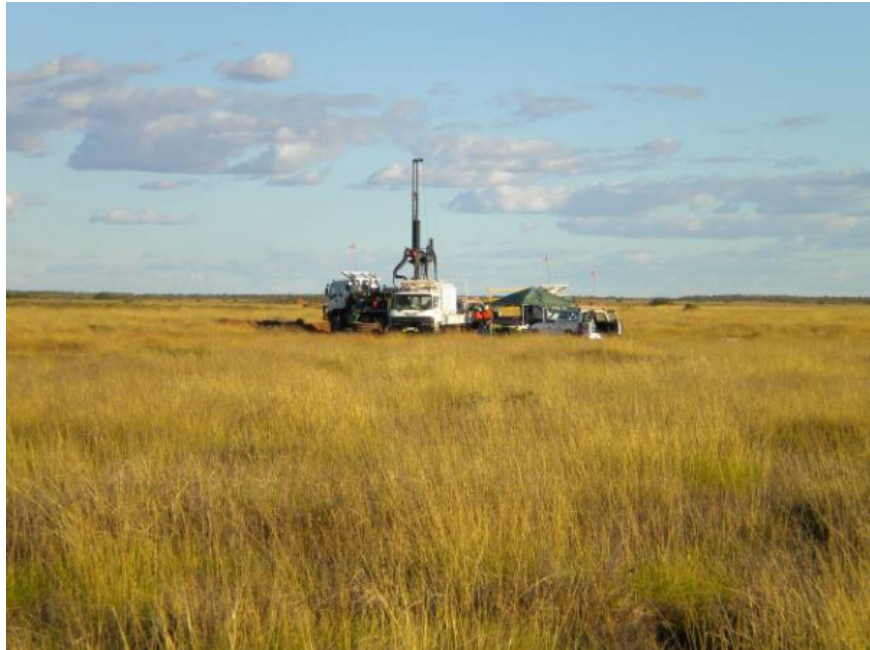
Photo # 1: Typical footprint of a geotechnical drilling rig at the Ashburton North site.
