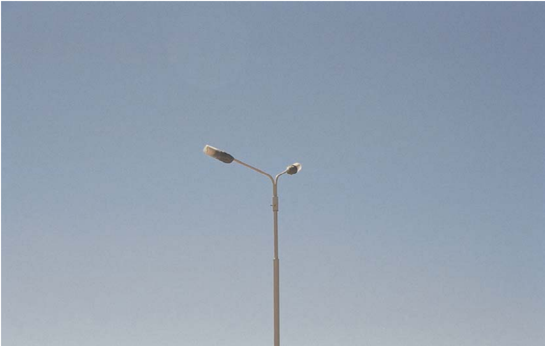
Plate 10: twin 80W sodium vapour street lights over camp parking lot.
