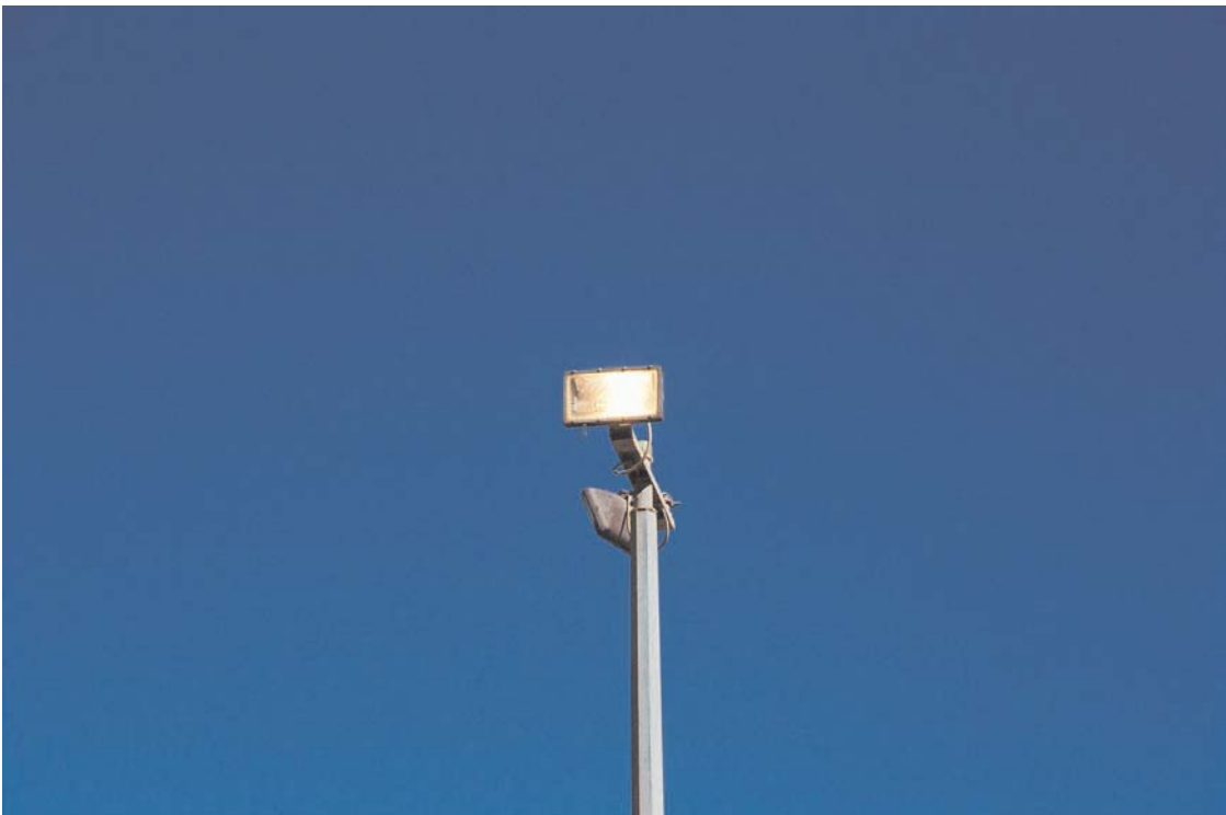
Plate 7: 400W sodium vapour light at the Terminal Tanks
